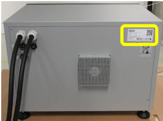
Figure 2-6: battery storage system, rear side
